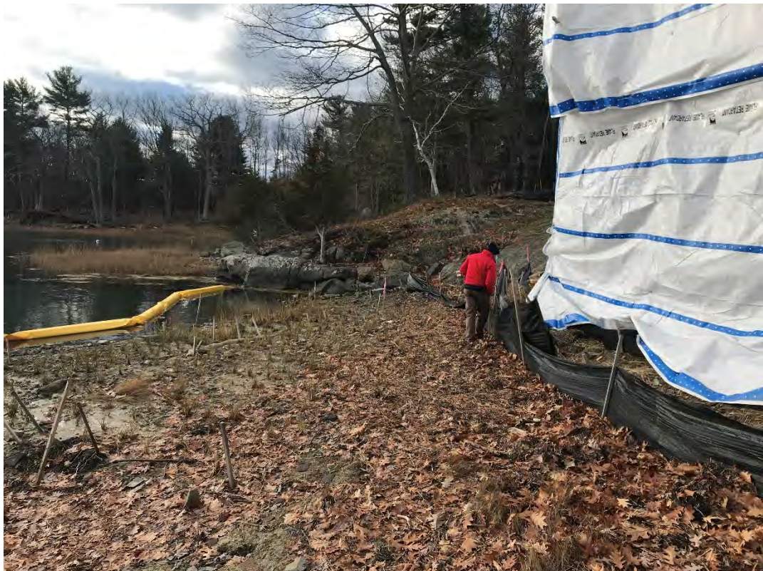
Fig 2: Toe of the slope and salt marsh restoration at the Eversource property/west side of the bay. Viewing south. (11-24-20)
