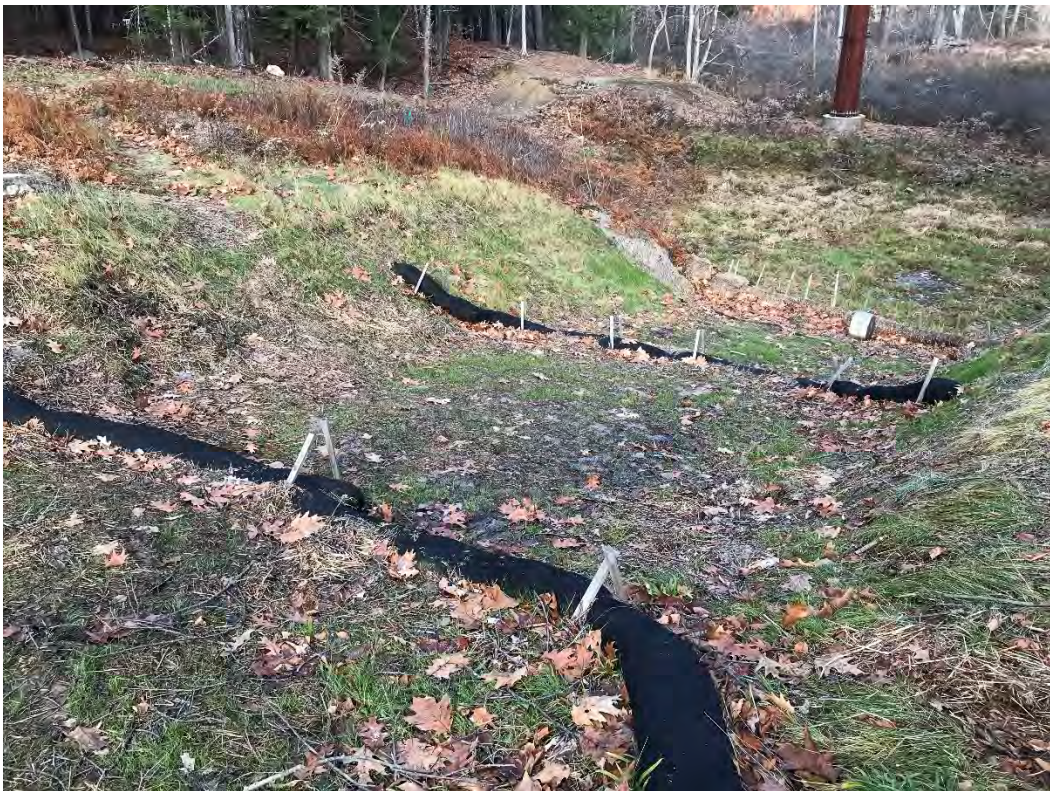
Fig 10: Slope between Strs. 28 and 29. Viewing north. (11-24-20)
